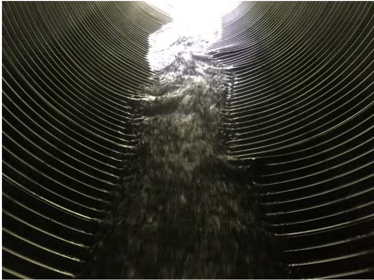
Minor damage noted on the floor
