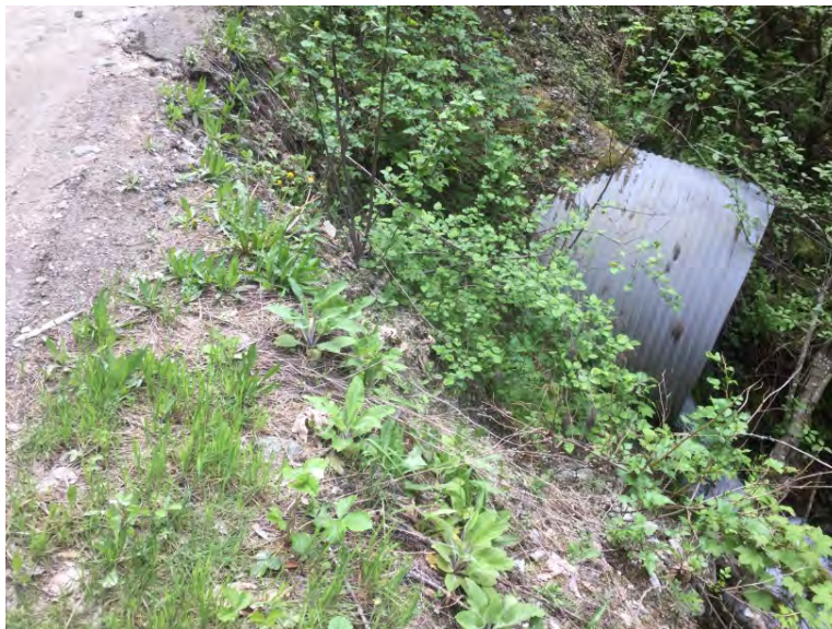
Fill erosion at downstream right bank
